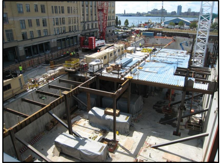
Figure 2: Photo of steel erection underway looking southwest. Photo taken by Vincent Rossi.
