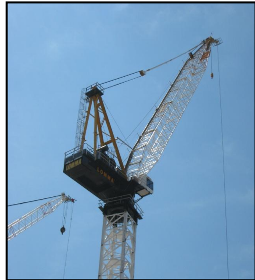
Figure 4: View of the tower crane on site. Photo taken by Vincent Rossi.
